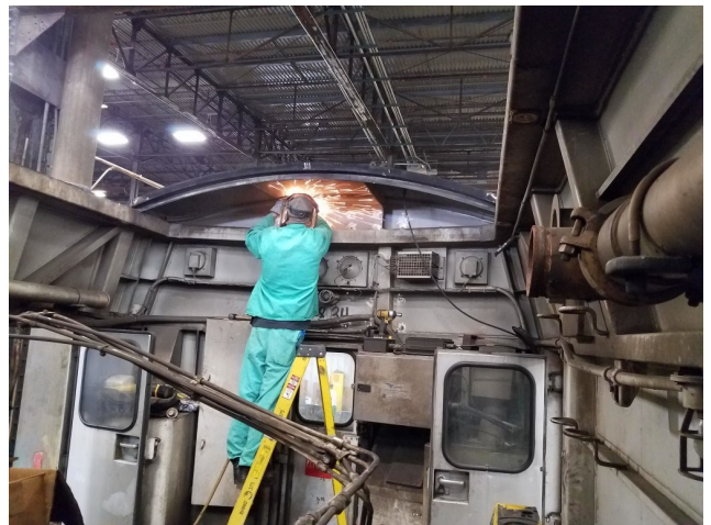
A worker in Amtrak's Beech Grove, Indiana facility works on a dismantled CTDOT P40 Locomotive
